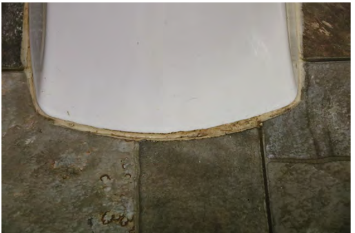
Dirty grout and caulking
