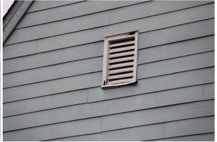
Frame of vent is disintegrating
