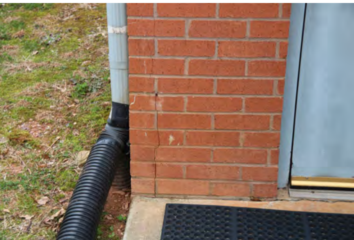
Significant crack at northwest corner of Parish Hall
