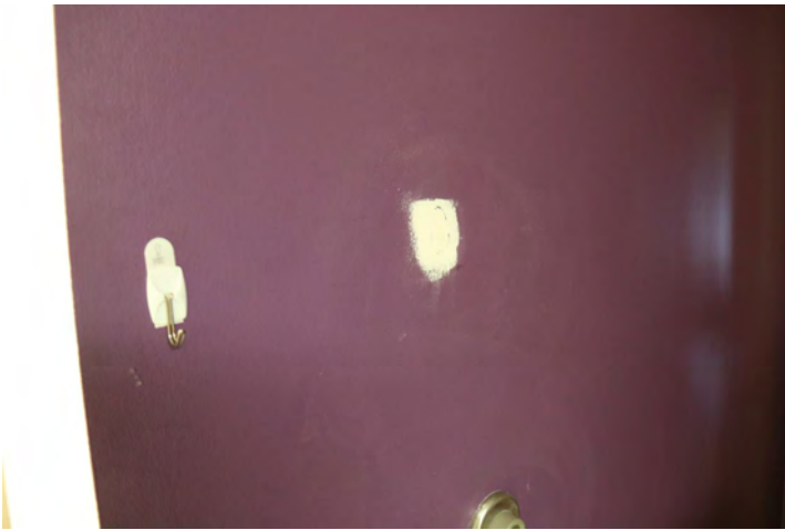
Incomplete wall repair
