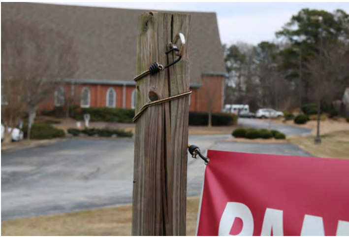
Sign posts are cracked and weathered
