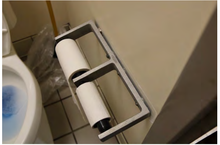
Toilet paper dispenser is coming loose from the wall
