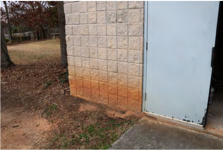
Soil accumulation on CMU walls
