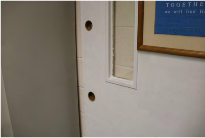
Missing door handle and lock
