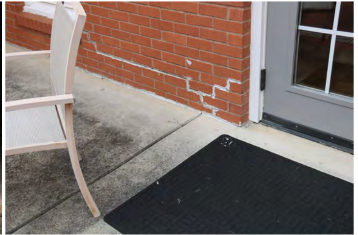
Inadequate repair of mortar joints
