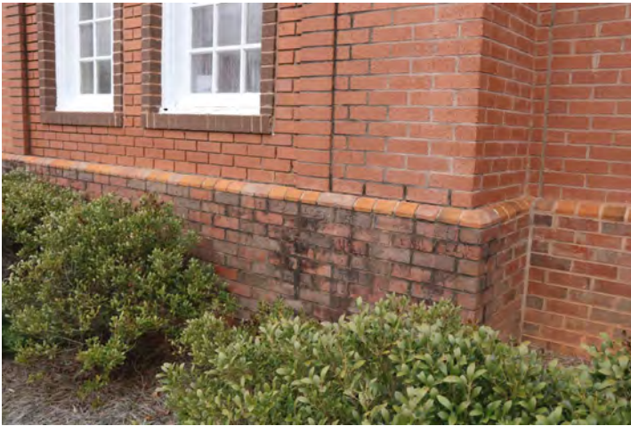
Accumulation of organic material on brickwork
