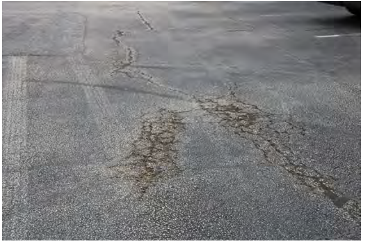
Repair areas of alligatoring
