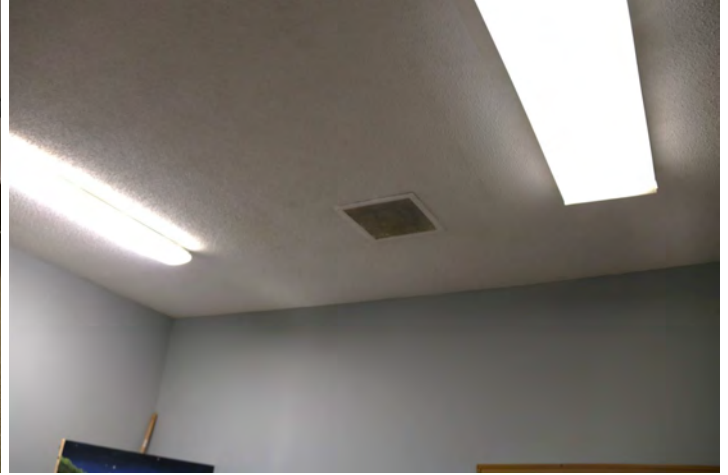
Ceiling vent in need of cleaning
