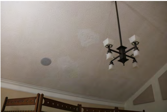
Mismatched ceiling repairs
