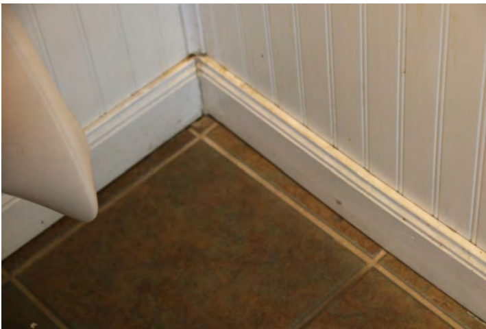
Accumulation of soil on base boards
