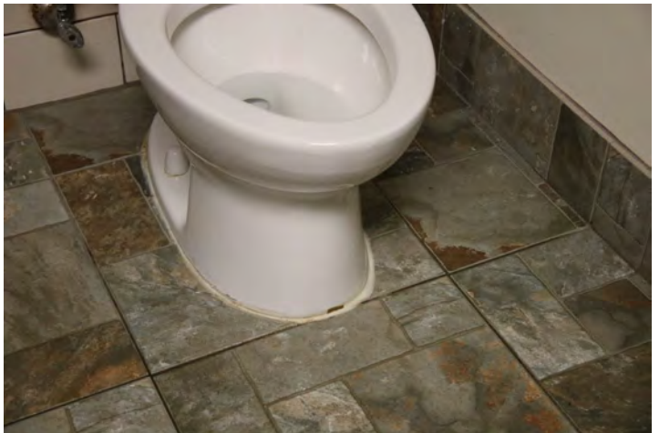
Dirty flooring and base of toilet
