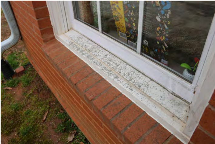
Organic growth on window frame
