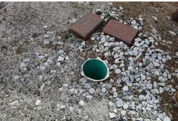
Replace drain cover
