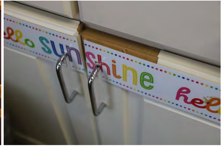
Damaged laminate on cupboard doors
