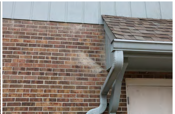
Discoloration of brickwork
