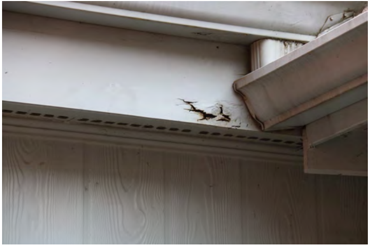
Deterioration of fascia possibly from overflowing gutter
