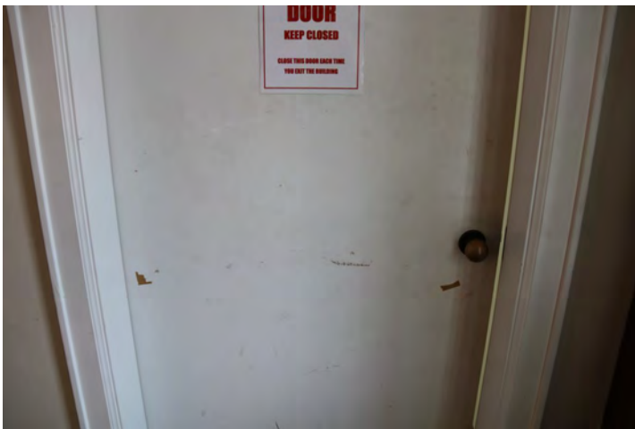
Dirty door with chipped paint
