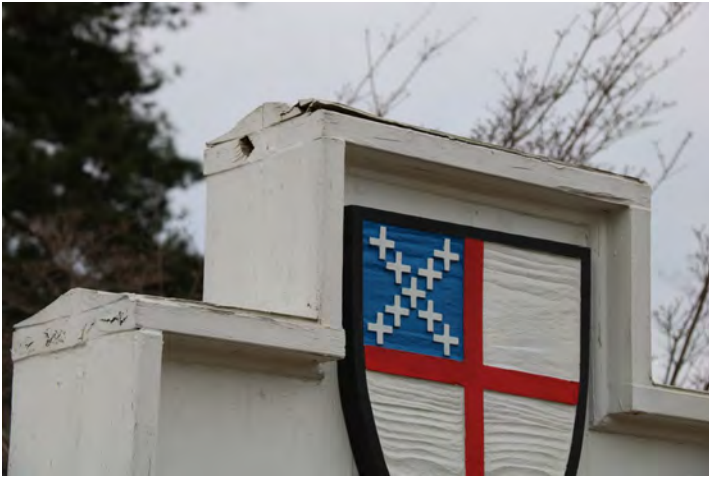
Wood trim on signage requires repair and repainting
