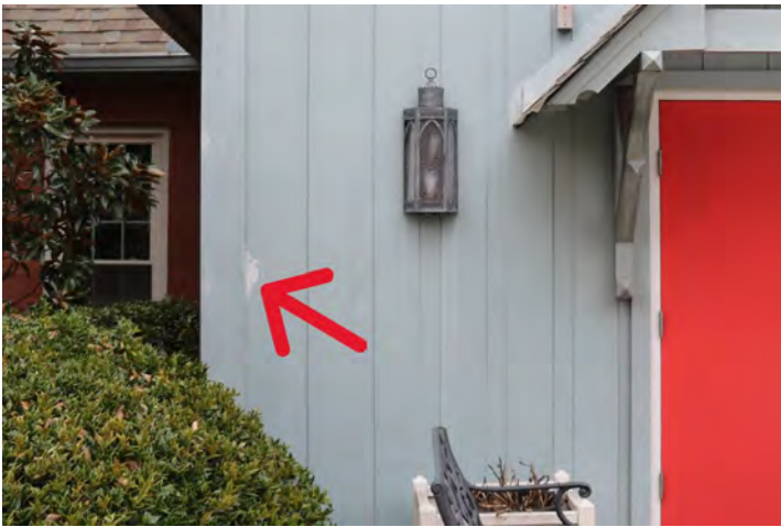
Incomplete repair requiring touch up paint
