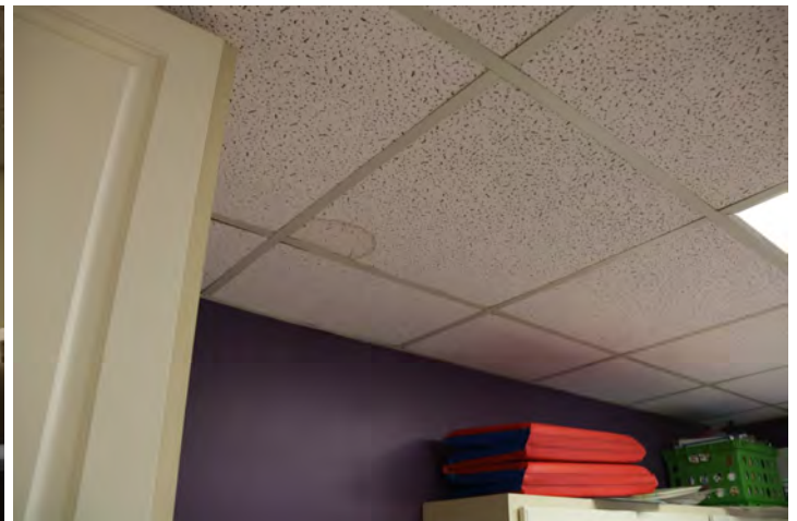
Stained ceiling tiles
