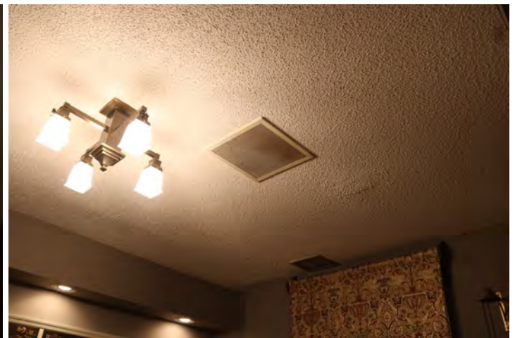
Regularly clean ceiling vents
