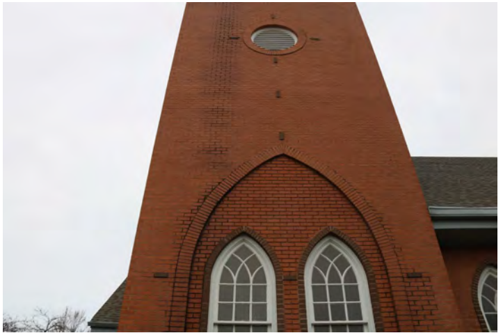
Bell tower shows signs of moisture retention mortar joint damage
