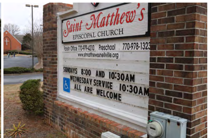
Signage displays buildup of soil and organic matter
