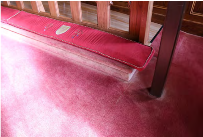
Discoloration of carpet likely due to inadequate vacuuming
