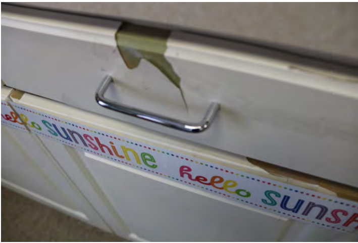
Broken laminate on drawer and door
