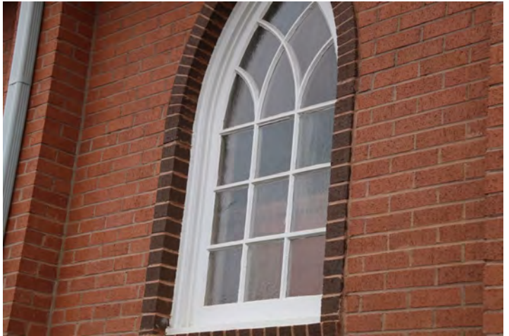
Sanctuary windows display compromised glazing
