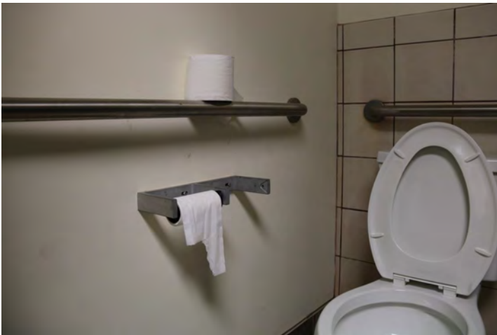
Missing roller on toilet paper dispenser
