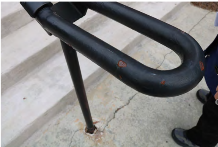
Rust on handrails
