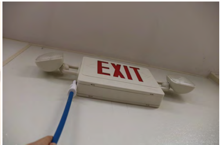
Emergency Exit light with failed back-up battery
