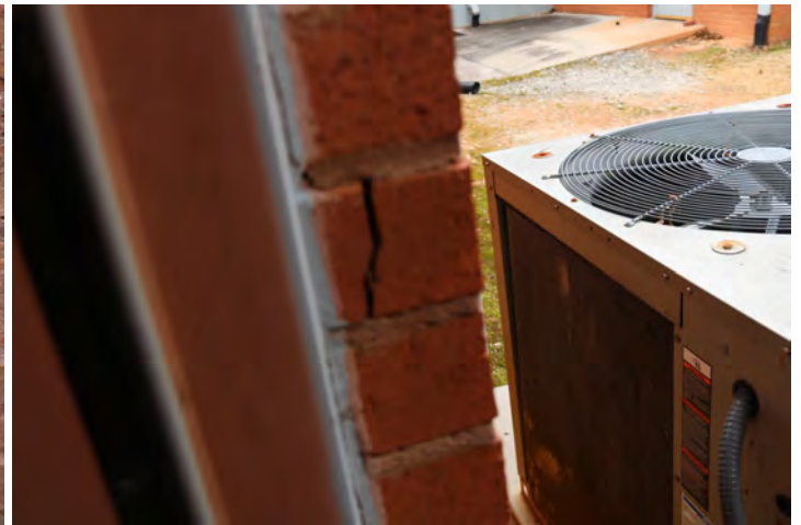
Crack in brick
