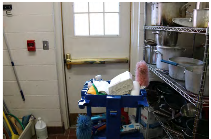
Emergency exit is obstructed
