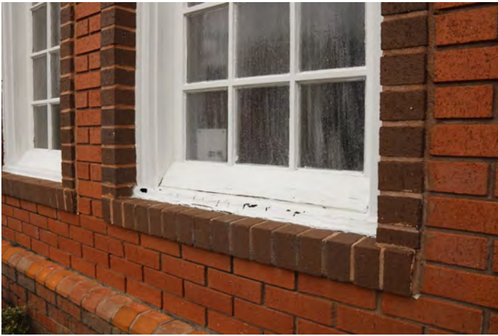
Deteriorating window frame
