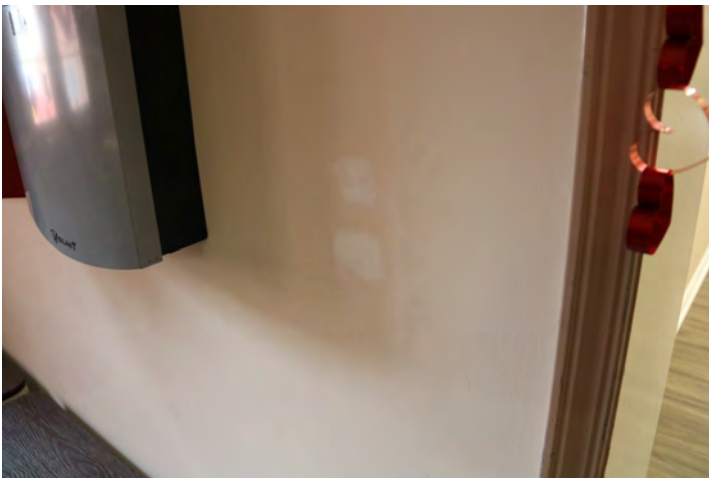
Incomplete wall repair
