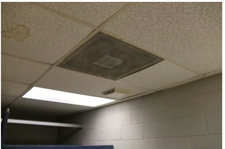
Stained ceiling tiles and dirty ceiling vents
