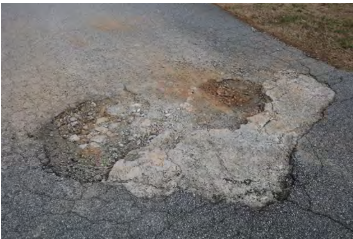
Repair areas with potholes
