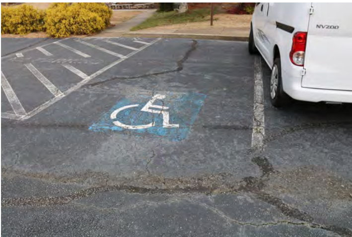
Painted ADA stall identification is fading
