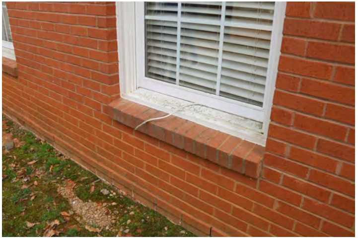
Damaged window seal
