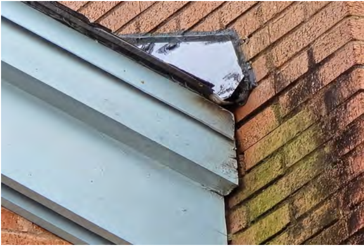
Deterioration on fascia and organic growth on masonry due to lack of roof drain
