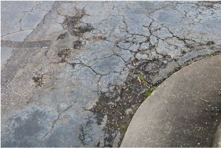
Repair compromised pavement at curbing
