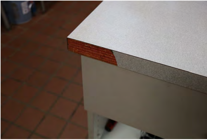
Broken laminate on counter edge
