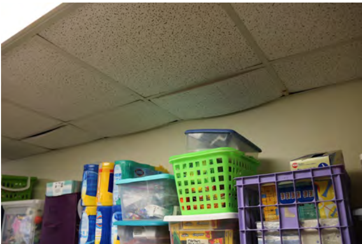
Ceiling tiles not firmly resting on grid
