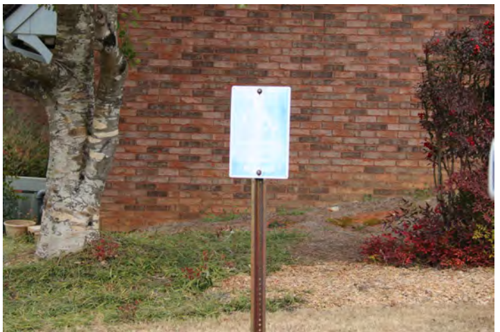
Faded ADA sign and rusted post
