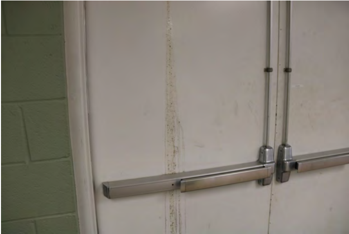
Cleaning door closer oil from door
