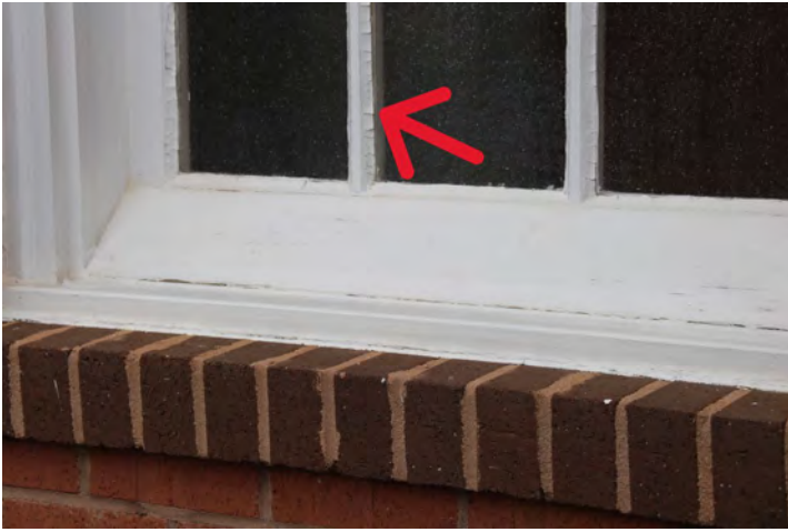
Compromised glazing putty
