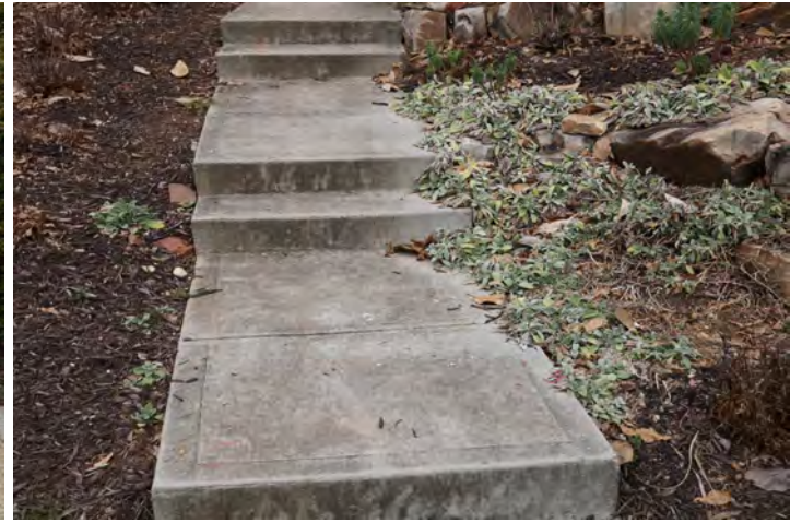
Trim vegetation back from walkway and step edges
