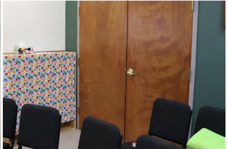
Scratched finish on doors
