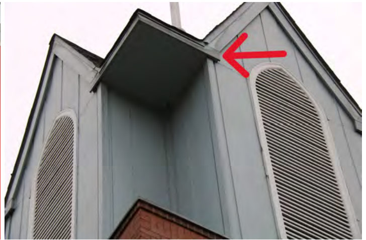
Worn and faded paint on fascia
