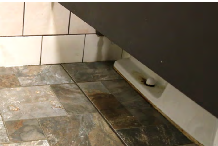
Dirty base of toilet and flooring
