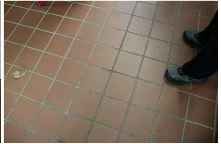
Dirty grout and floor tile
