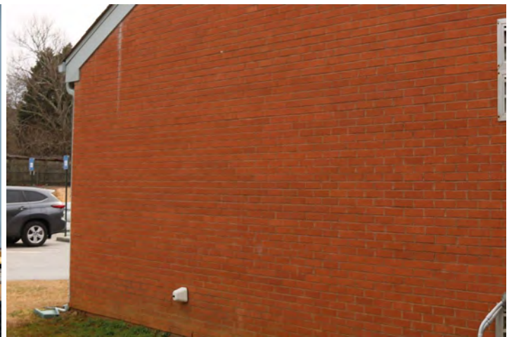
Stain and accumulated soil on brickwork
