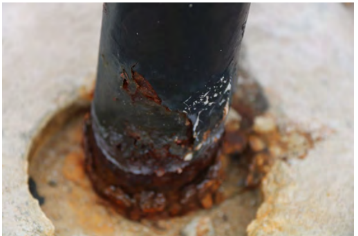
Replace handrail portions with significant rust
