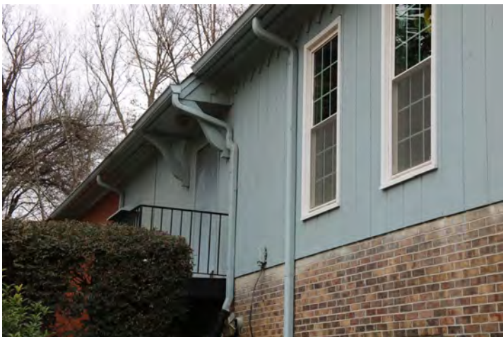
Brickwork exhibits discoloration beneath siding
