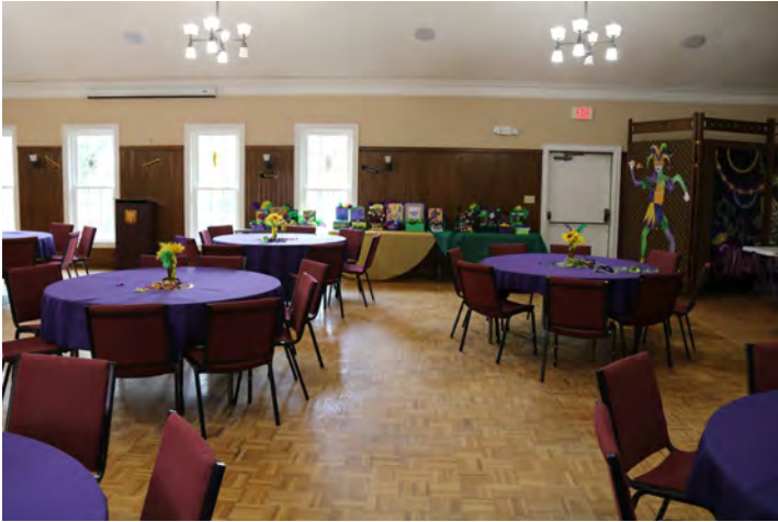
Parquet flooring appears worn and dull
