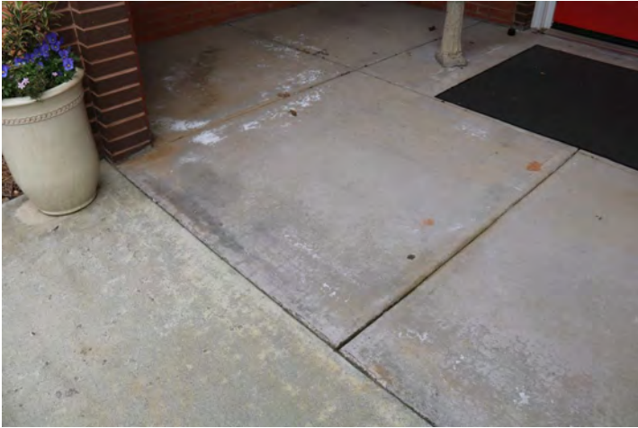
Clean ice melt residue to prevent spalling
