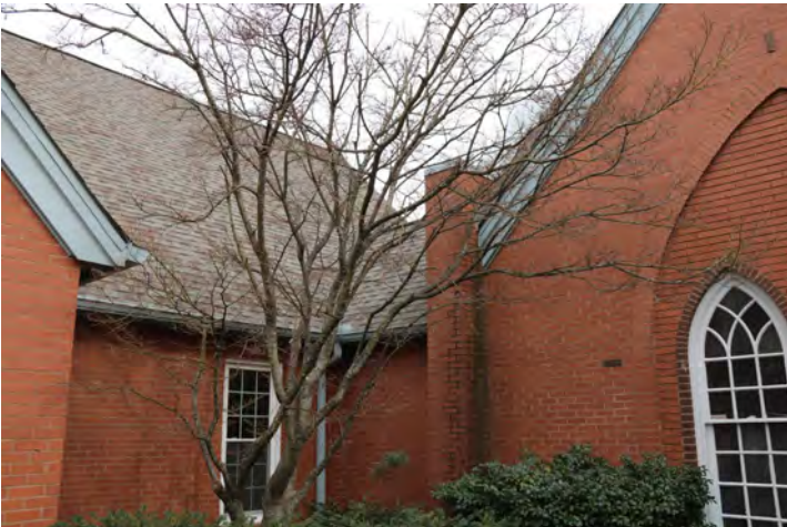
Trim tree branches back away from walls and roof areas
