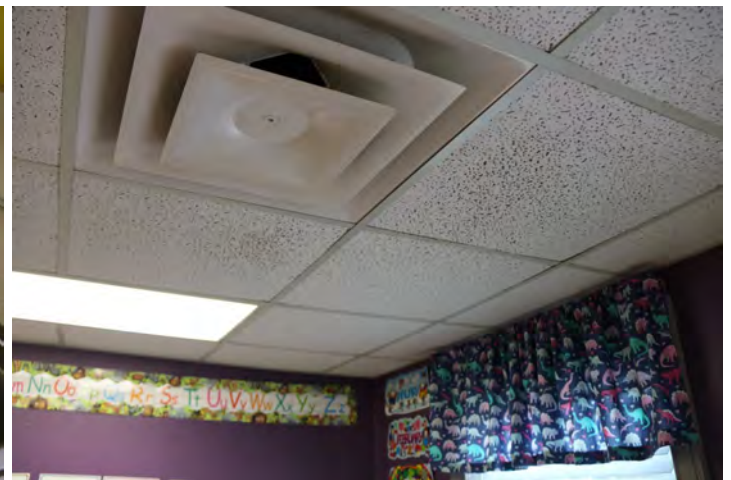
Dirty ceiling vent and tiles
