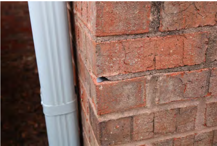
Compromised mortar joints and cracked bricks
