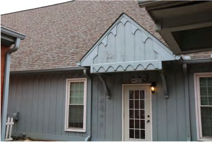
Siding shows soil accumulation and peeling paint
