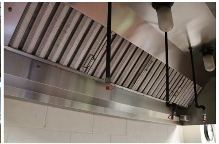
Vent hood in need of deep cleaning
