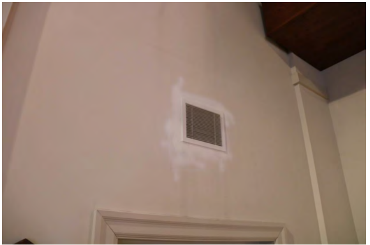
Incomplete wall repair
