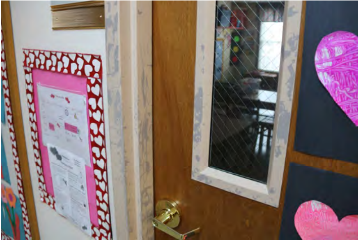
Peeling paint on door and relite frames
