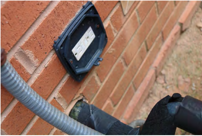
Ensure all exterior outlets have weatherproof covers
