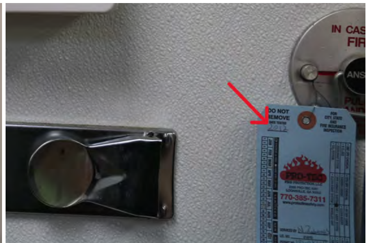
ANSUL fire suppression last inspected in 2012
