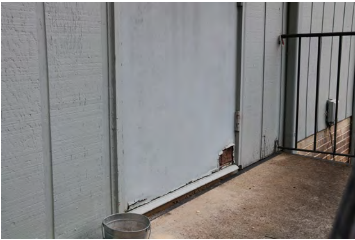
Replace deteriorated door
