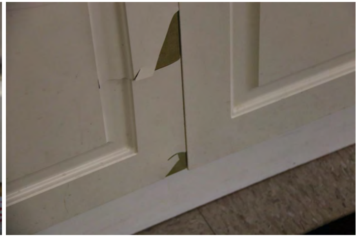
Broken laminate on cupboard doors
