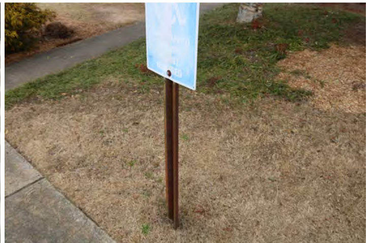
ADA signage is faded and sign post is rusted
