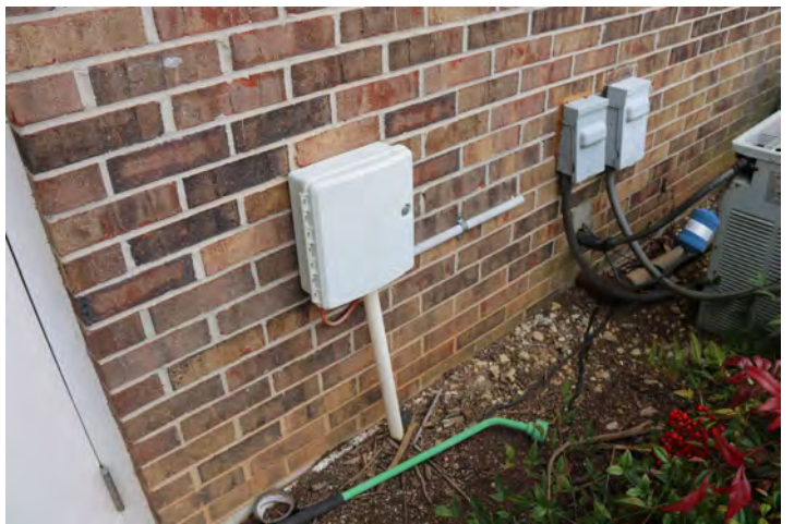
Repair non-functioning irrigation system
