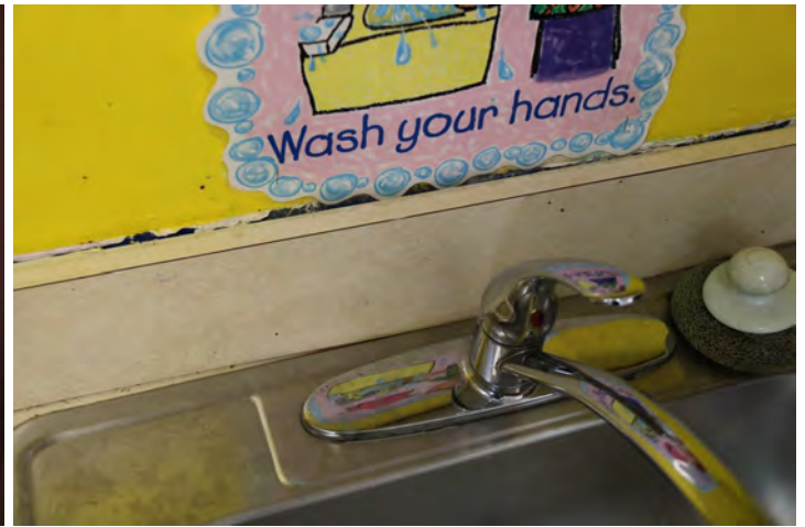
Dirty sink area and splash panel is coming loose from wall
