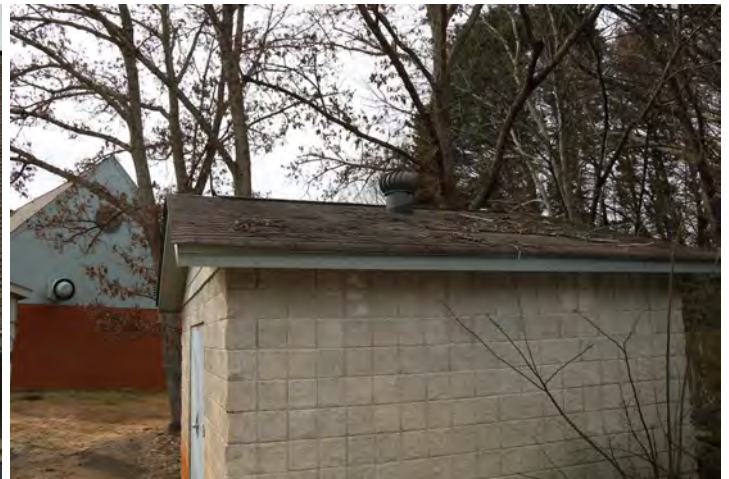
Remove debris and consider adding gutters
