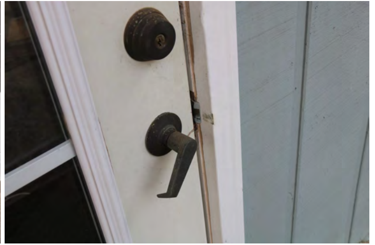
Replace damaged handset hardware
