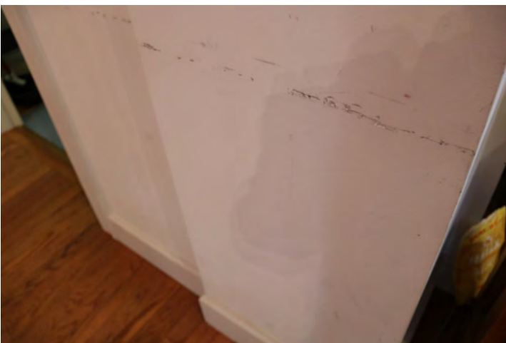
Wall damage in need of patching and painting
