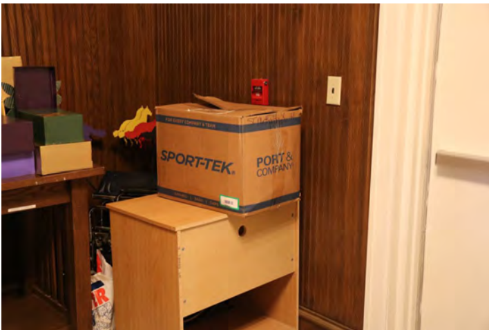
Fire pull station is obstructed
